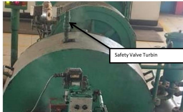
Gambar 2.16 Safety Valve Turbin (Adibrata Unggul Jaya)
