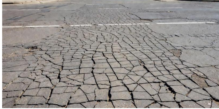
Gambar 2.4 Retak Buaya (FHWA, Distress Identification Manual)
