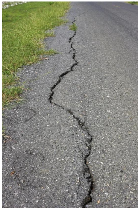
Gambar 2.5 Retak Pinggir (FHWA, Distress Identification Manual)
