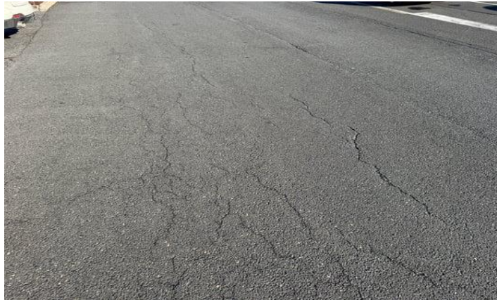
Gambar 2.3 retak rambut (FHWA, Distress Identification Manual)
