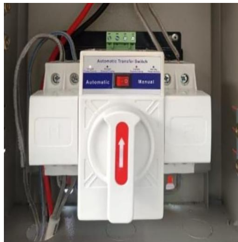
Gambar 3. 6 ATS (Auto Transfer Switch)
