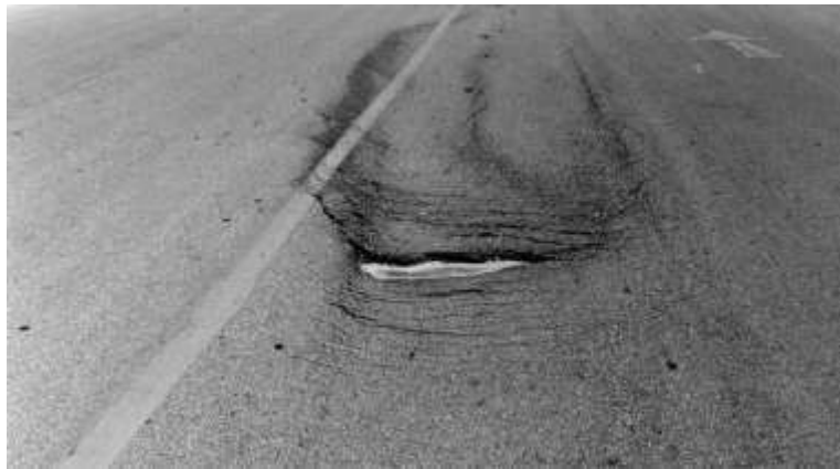
Gambar 2.21: Retak Slip ( Slippage Cracking )
