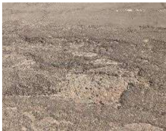
Gambar 2.22: Pelapukan dan butiran lepas ( Weathering and Raveling )
