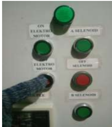
Gambar 4.23 Push Button Off Elektro Motor
