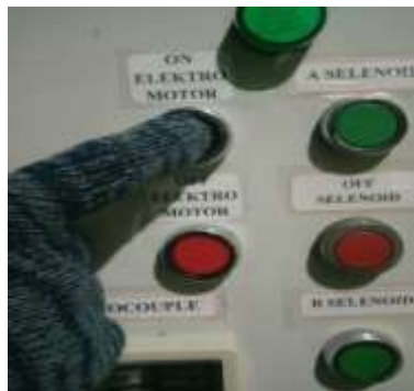
Gambar 4.19 Push Button On Elektro Motor
