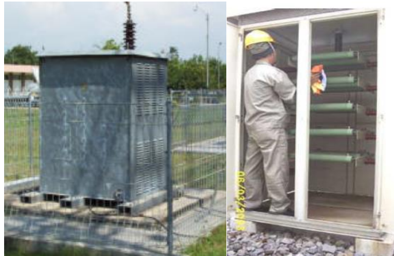
Gambar 2.11 Neutral Grounding Resistor (NGR)
