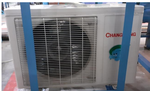
Gambar 3.2 Unit Outdoor AC Split
