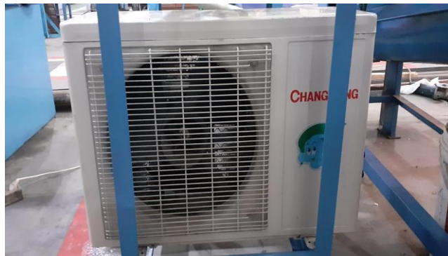
Gambar 3.3. Unit Outdoor AC Split
