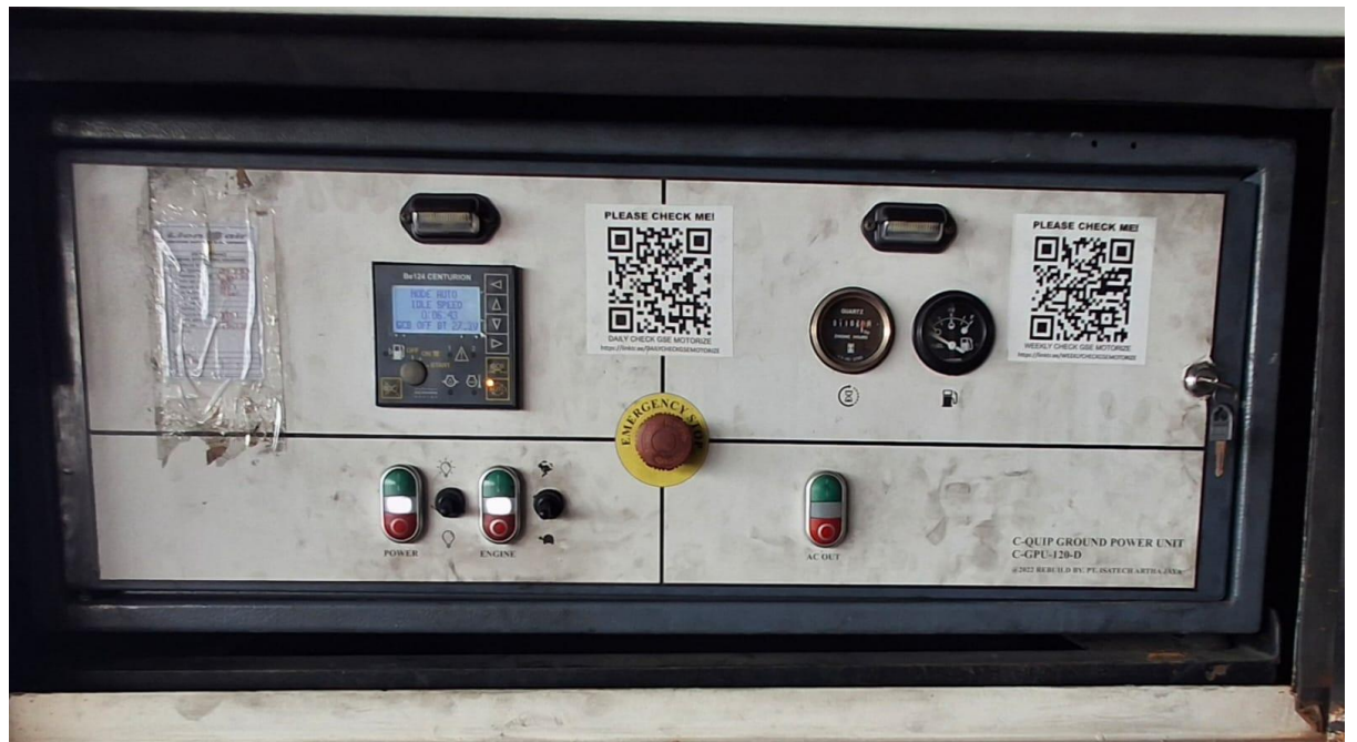
GBR. PANEL CONTROL GPU
