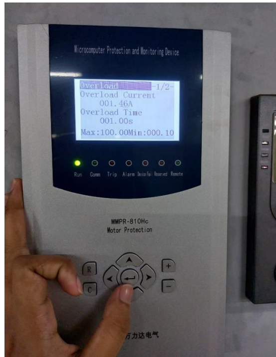
Gambar 4.9 Microcontroller Motor Protection Relay
