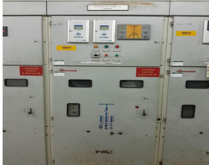
Gambar 4.7 Panel Motor 6kv (1A) Boiler Feed Water Pump
