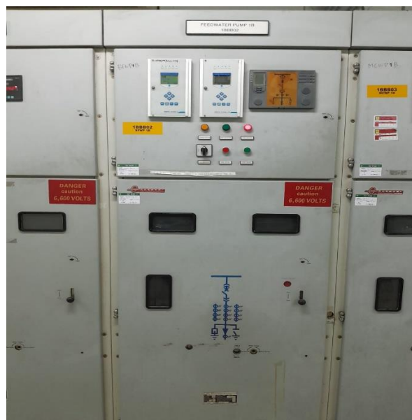
Gambar 4.6 Panel Motor 6kv (1B) Boiler Feed Water Pump
