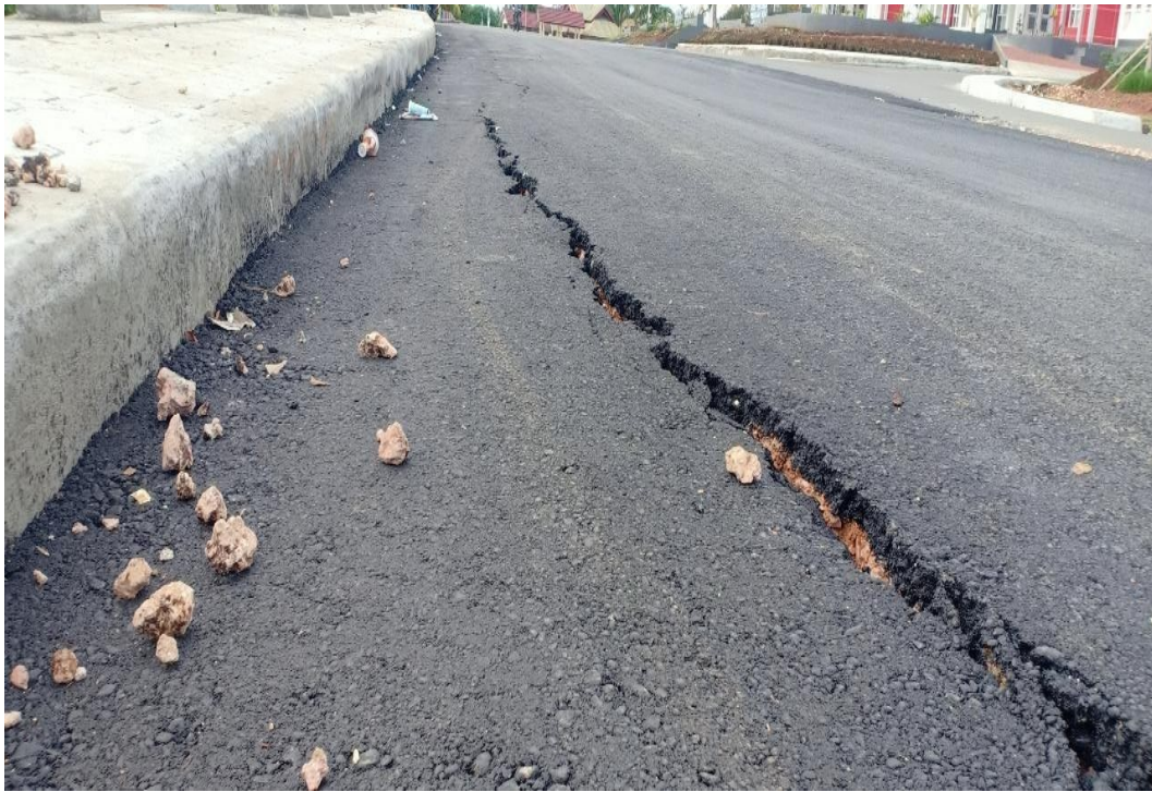
Gambar 2.8: Retak Sambung ( Joint Reflect Cracking ).
