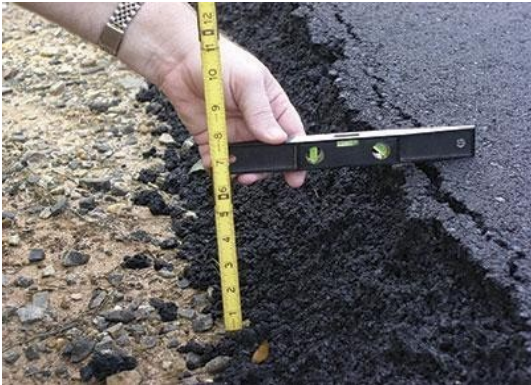
Gambar 2.9: Pinggiran Jalan Turun Vertikal ( Lane/ Shoulder Drop Off ) Sumber: https://www.pikiranlampung.com/2022/11/ketebalan-aspal-jalan-poros-di-waway.html
