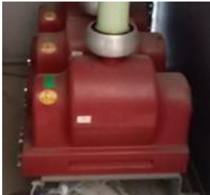
Gambar 2.8 Trafo Tegangan (Potensial Transformer)
