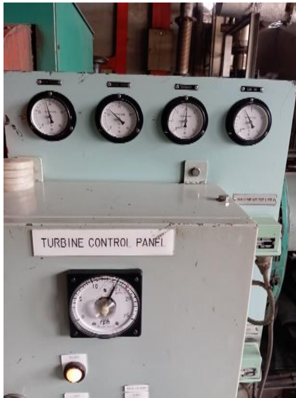
Gambar 3.4 Turbin Control Panel
