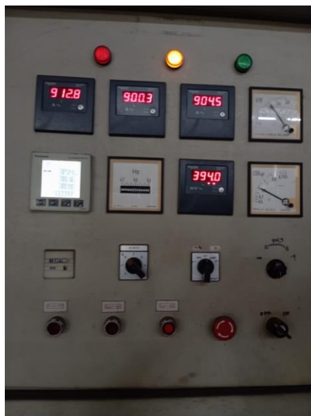
Gambar 3.3 Control Panel Turbine
