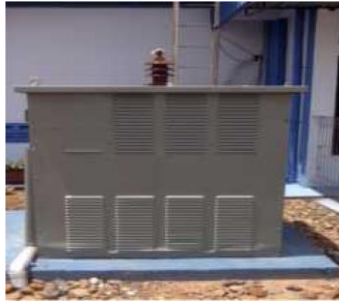
Gambar 2.4 Neutral Grounding Resistance
