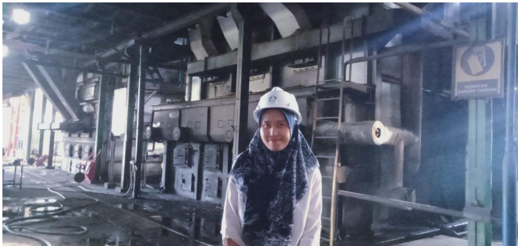
Boiler Takuma N1000 Kapasitas 35 ton Uap/jam
