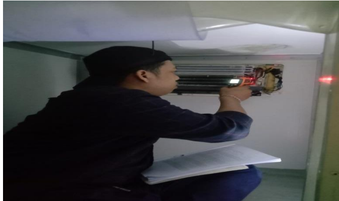
Gambar 4.4 Pengukuran suhu pipa evaporator
