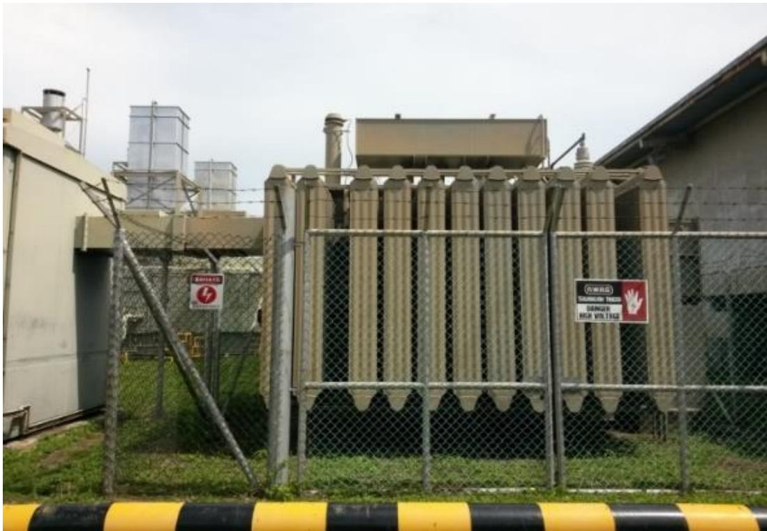
Gambar 2.1. Transformator daya PT. Perta Arun Gas Lhokseumawe
