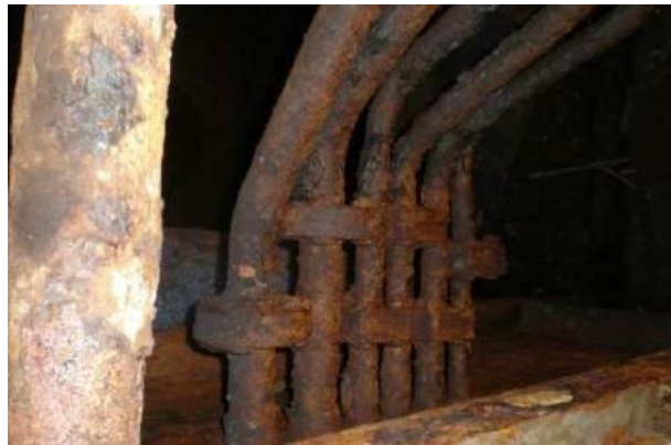
Gambar 2.5 Korosi Seragam Pada Pipa Ballast (Pattireuw Kevin J,2013)
