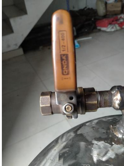
Gambar 4.13 katub uap ( steam valve )
