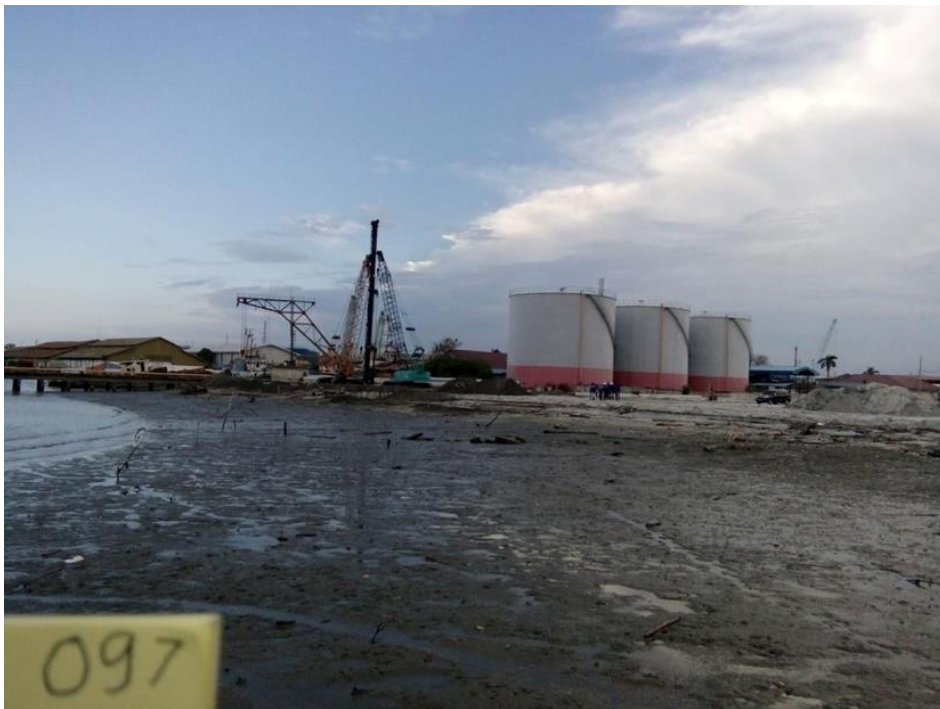
Lampiran 1. 8 Kondisi Marking 097
