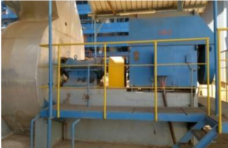
Gambar 2.11. Induced Draught Fan
