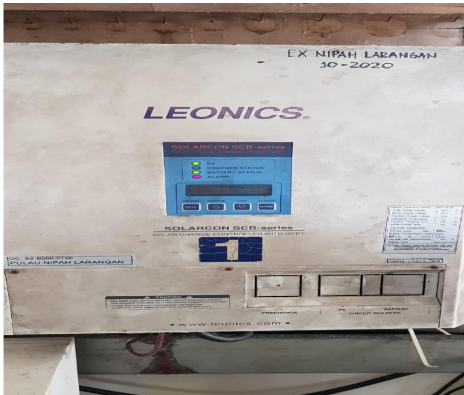
Maximum Power Poin Trecking (MPPT)
