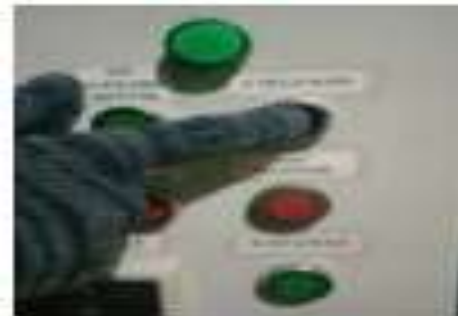
Gambar 4.19 Push Button On Elektro Motor
