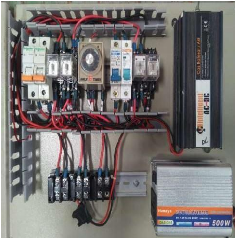
Gambar 4.1 Panel Back-Up Power
