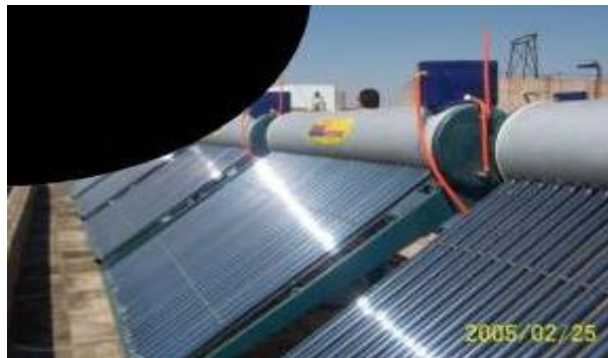
Gambar 2.5 Solar Water Heater
