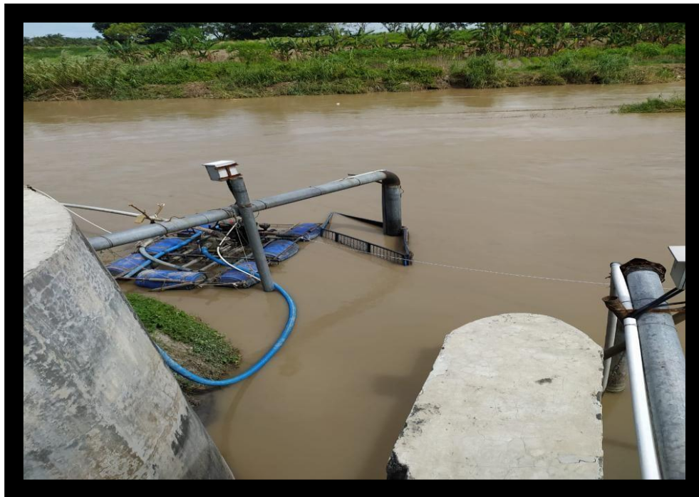
Gambar 1.4: Intake sumber air PDAM Tirta Bina
