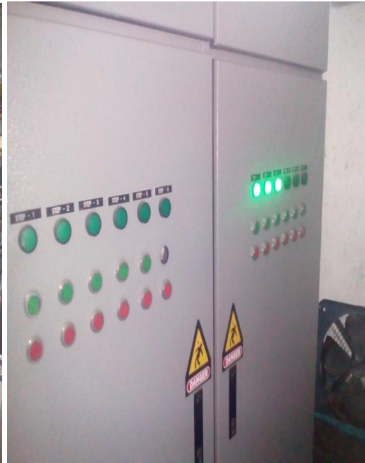
Gambar Panel Box Kapasitor Bank
