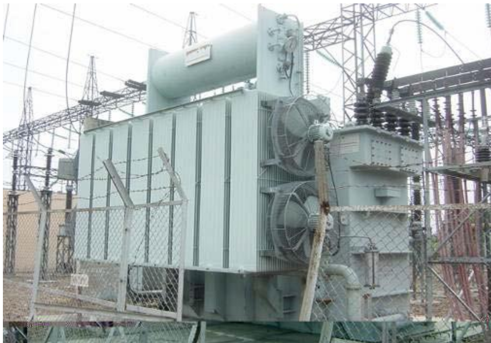
Gambar 3.1 Transformator Daya 1 (TD 1)
