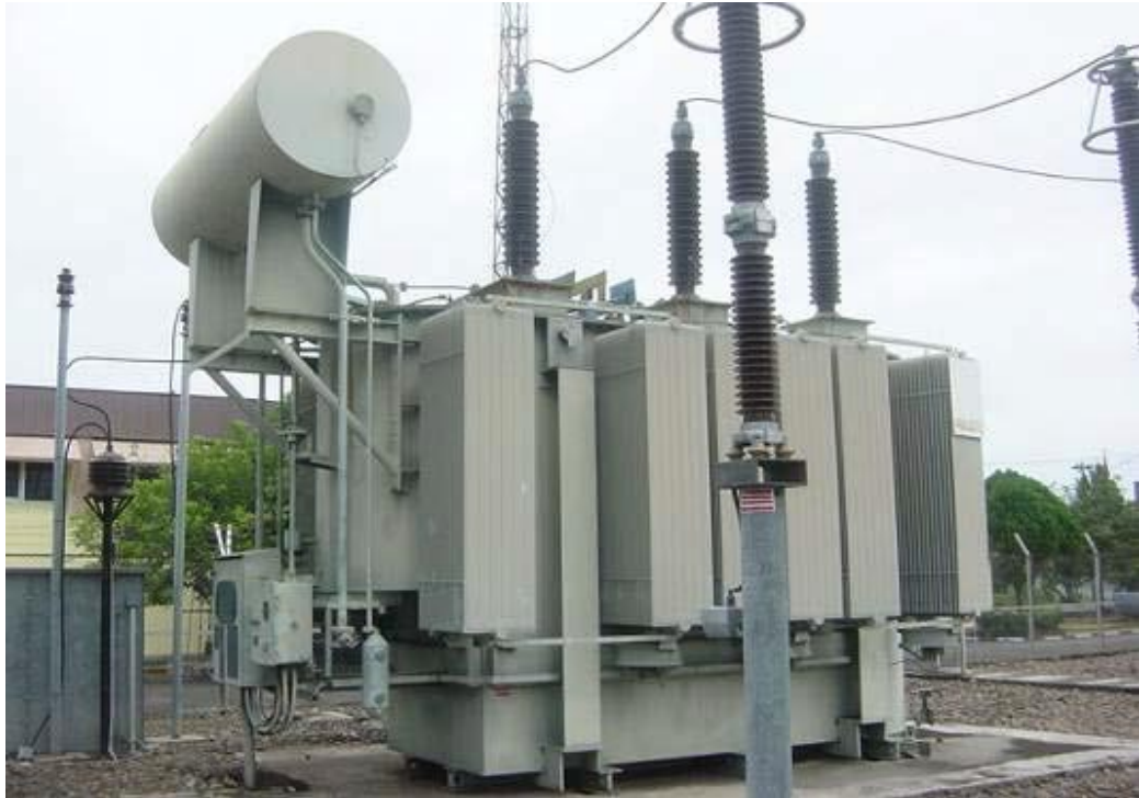
Gambar 3.2 Transformator Daya 3(TD 3)
