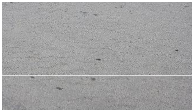
Gambar 2.3: Retak rambut ( Hair Cracks ) (SOP PUPR 2016).
