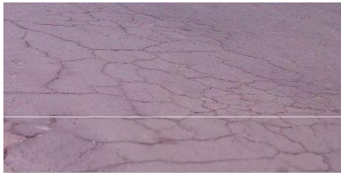
Gambar 2.4: Retak kulit buaya ( Alligator Cracks ) (SOP PUPR 2016).
