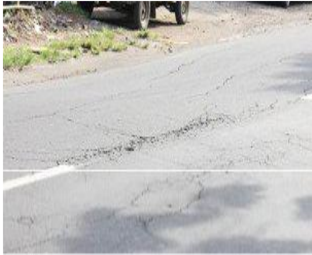
Gambar 2.6: Retak sambungan jalan ( Lane Joint Cracks ) (SOP PUPR 2016).
