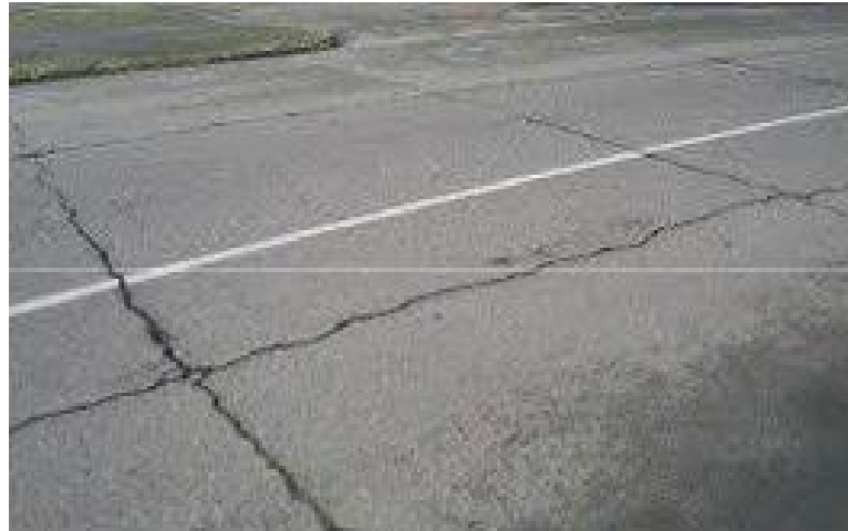
Gambar 2.8: Retak refleksi ( Reflection Cracks ) (SOP PUPR 2016).
