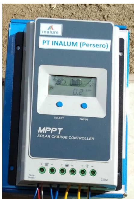
Gambar 2.6 MPPT (Maximum Power Point Tracking)
