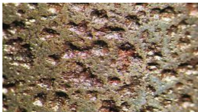
Gambar 2.7 Korosi Sumuran (Pitting Corrosion)
