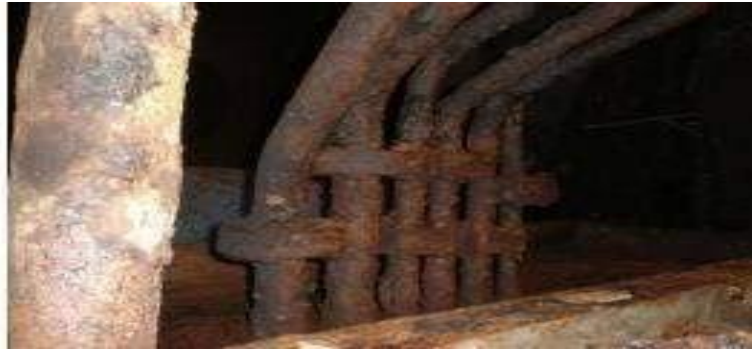
Gambar 2.4 Korosi Seragam (Uniform Corrosion)
