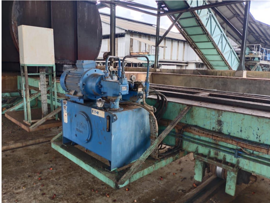
Gambar 2. 4 HPU ( Hidrolic Power Unit)
