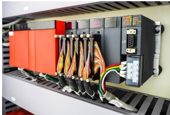
Gambar 2. 16 PLC (programmable logic control)
