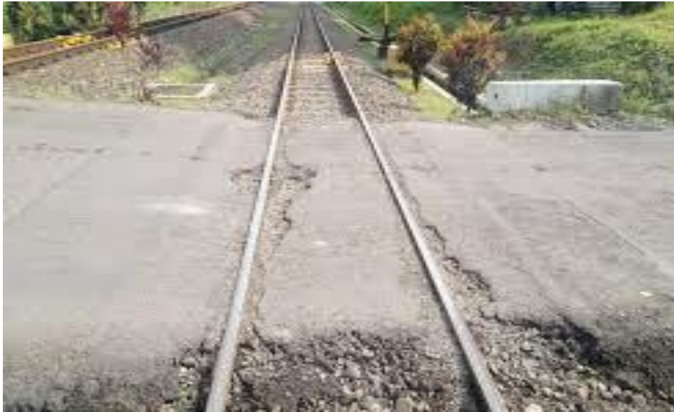
Gambar 2.18: rusak perpotongan rel/ railroad cracking (google)
