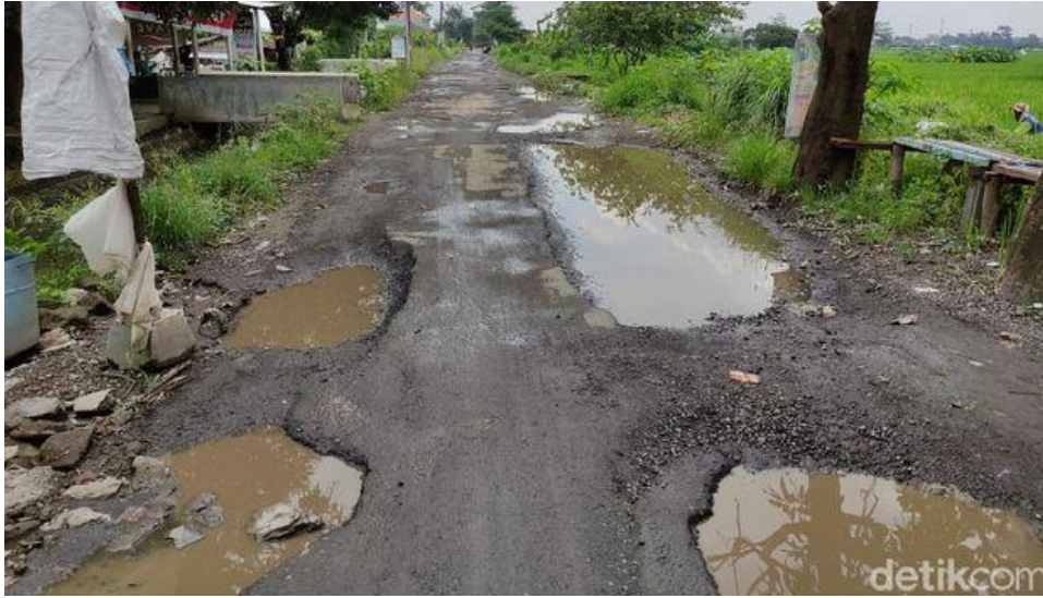
Gambar 2.17: lubang/ pothole (google)
