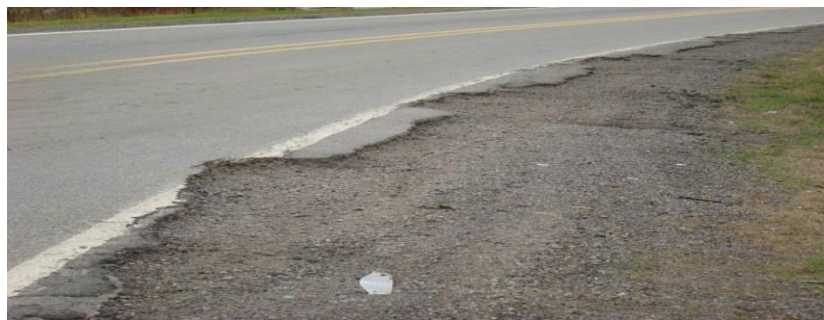
Gambar 2.13: pinggiran jalan turun vertical/ line shoulder drop (google)
