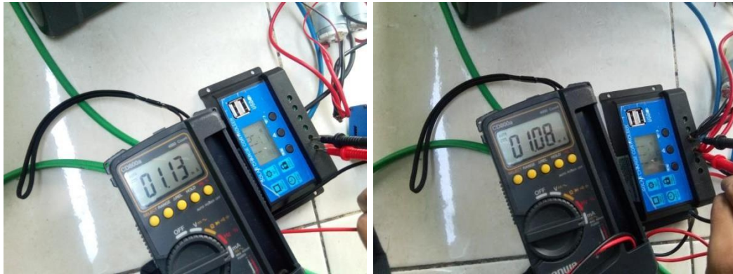
Gambar 4.18 V_{in} , I_{in} SCC & V_{out} , I_{out} SCC
