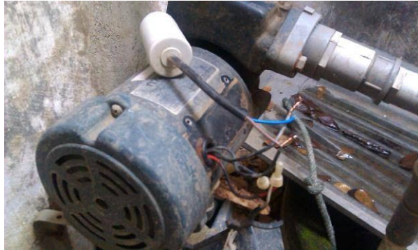
Gambar 3. Motor pompa air 1phase
