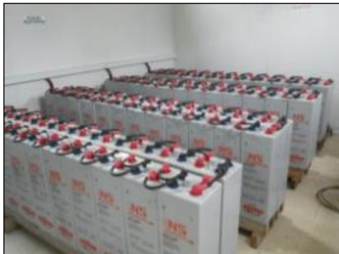
Gambar 2.10 Energy Storage (baterai)[24]
