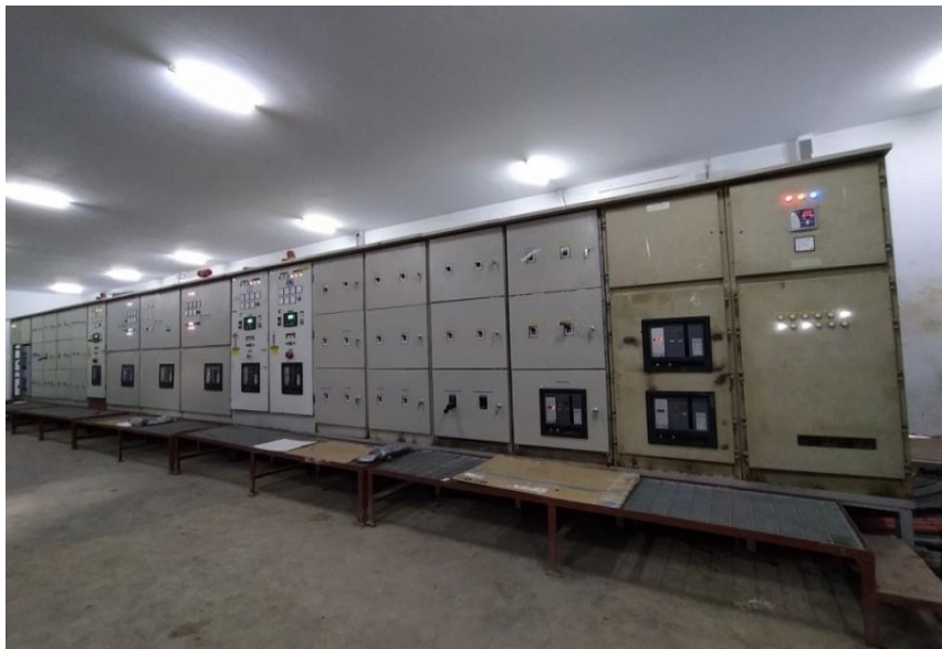
Gambar 3.1 Main Switch Board (MSB)
