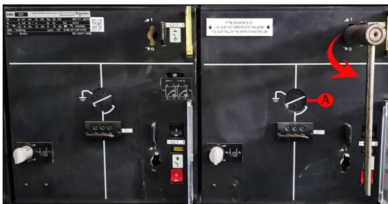
Gambar 3.10 Status DS ( disconnecting switch ) open
