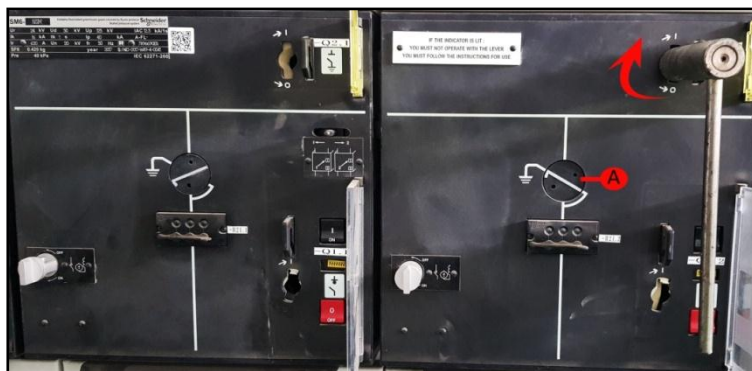
Gambar 3.9 Status Earthing switch
