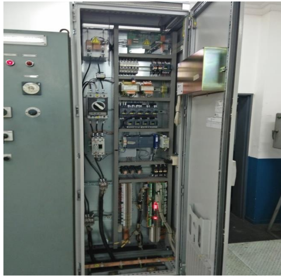
Gambar 3.2 Control Cabinet FL SMIDTH
