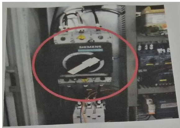
Gambar 3.5 MCB Panel Trafo.
