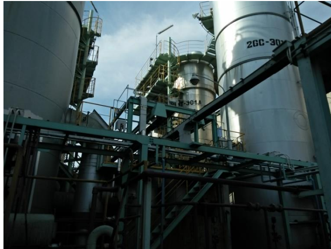
Gambar 3.3 Station Gas 4DT – 301B
