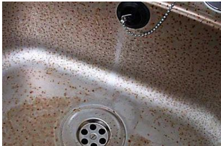
Gambar 2.3 Korosi Lubang ( Pitting ) (Utomo, 2012)
