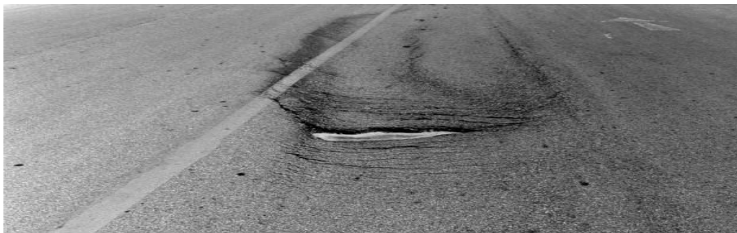
Gambar 2. 9 : Retak Slip (Slippage Cracks) (dpu.kulonprogokab n.d.)
