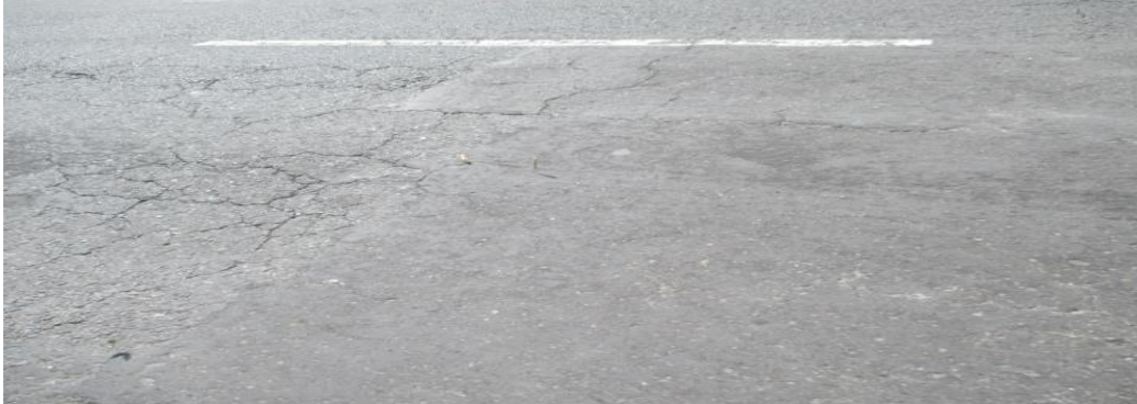
Gambar 2. 2 : Retak Halus (Hair Cracking) (dpu.kulonprogokab n.d.)
