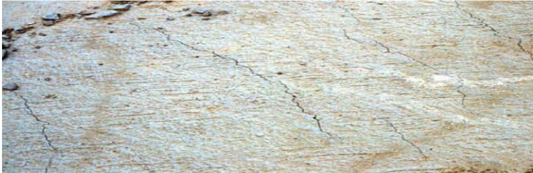
Gambar 2. 8 Retak Susut (Shrinkage Cracks) (dpu.kulonprogokab n.d.)
