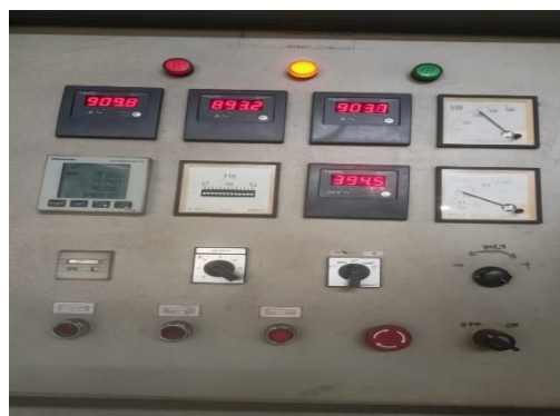
Gambar 3.5 Control Panel Turbine
