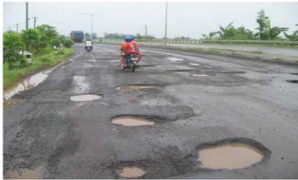
Gambar 2.12: Kerusakan lubang ( potholes ) (Hardiyatmo, 2015).
