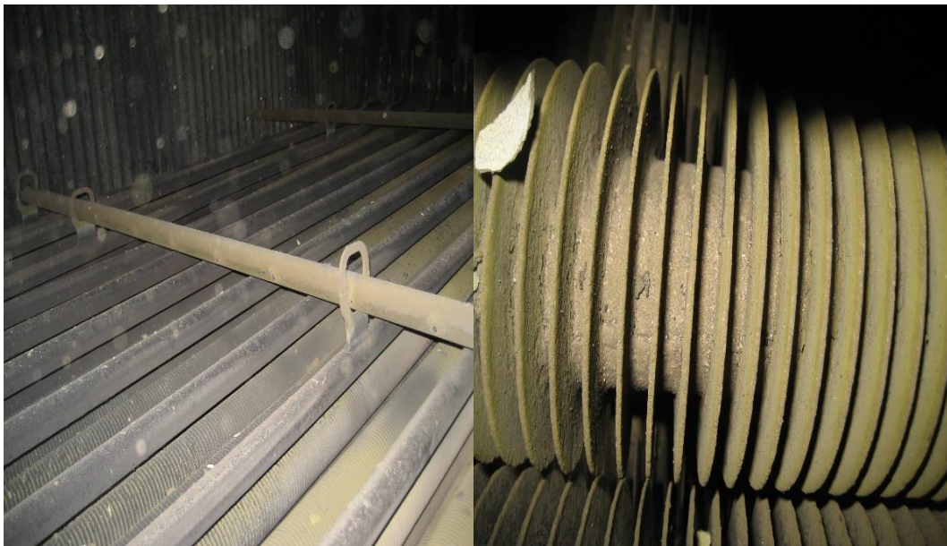
Gambar 4.6 Tube-tube economizer sisi atas ( Outlet feedwater )
