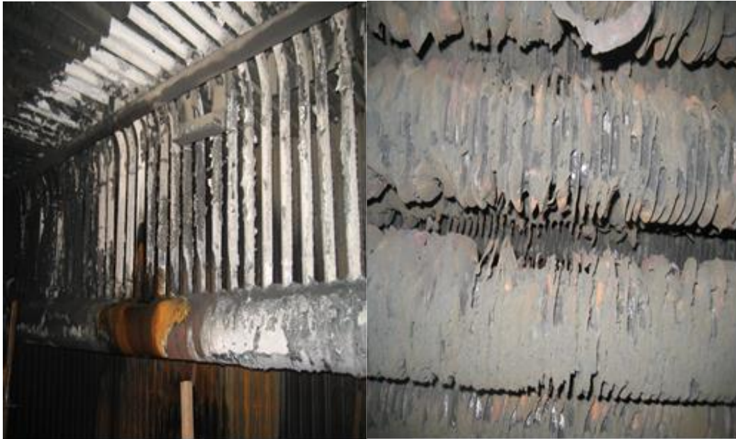
Gambar 4.7 Tube-tube header economizer (sisi bawah/inlet feedwater)
