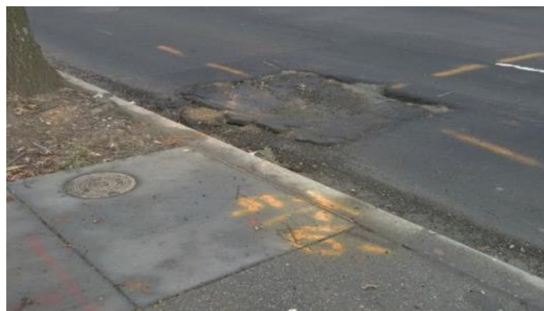
Gambar 2.16. Utility Cut Depression Sumber : Dinas PUPR Kulonprogo (2021)
