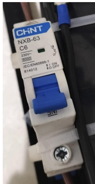
Gambar 3.4 Miniature Circuit Breaker (MCB)
