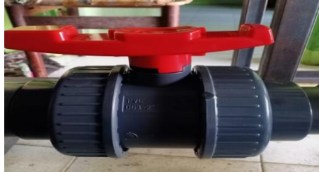
Gambar 3.39 Kran Air ( Valve )
