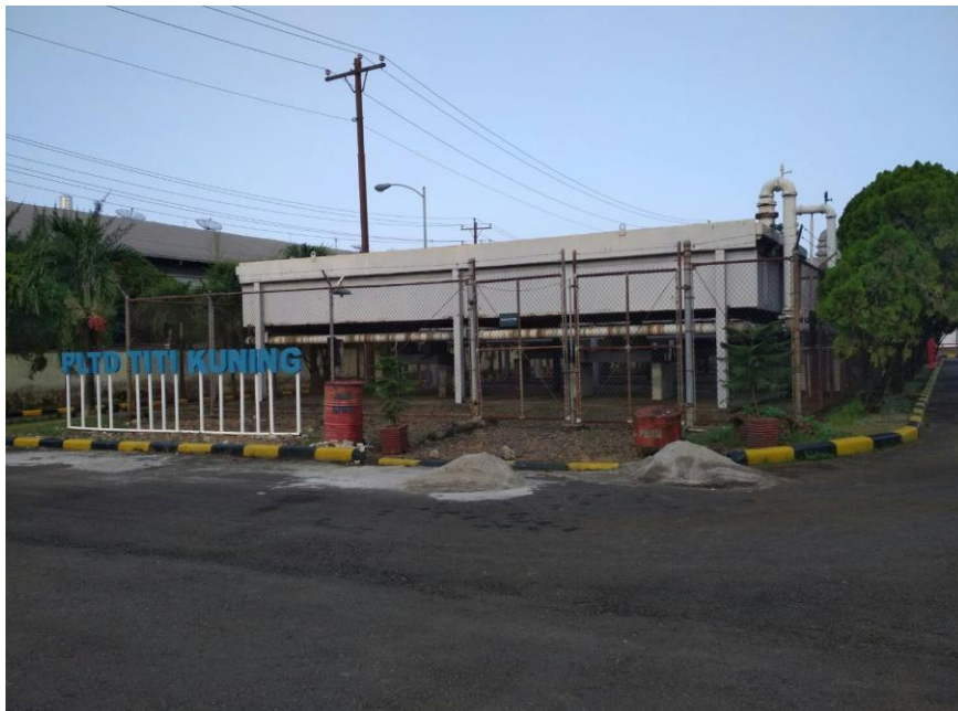
GAMBAR RADIATOR PEMBANGKIT LISTRIK TENAGA DIESEL TITI KUNING.
