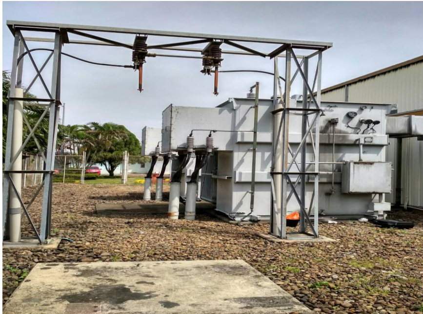
GAMBAR TRANSFORMATOR DAYA (STEP UP) PEMBANGKIT LISTRIK TENAGA DIESEL TITI KUNING.
