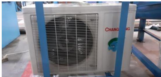
Gambar 3.6 Unit Outdoor AC Split
