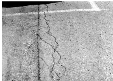
FIG. X1.20 Medium-Severity Edge Cracking
