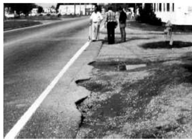
FIG. X1.21 High-Severity Edge Cracking
