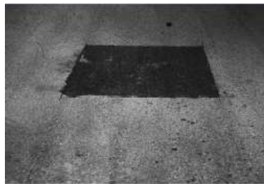
FIG. X1.31 Low-Severity Patching and Utility Cut Patching
