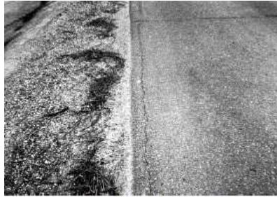
FIG. X1.19 Low-Severity Edge Cracking
