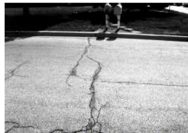
FIG. X1.8 Medium-Severity Block Cracking
