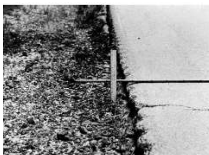
FIG. X1.27 High-Severity Lane/Shoulder Drop-Off
