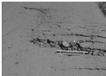
FIG. X1.49 High-Severity Slippage Cracking
