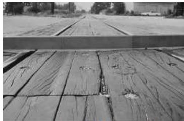
FIG. X1.38 Low-Severity Railroad Crossing
