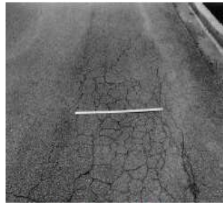
FIG. X1.2 Medium-Severity Alligator Cracking
