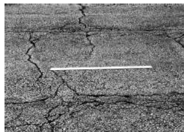
FIG. X1.7 Low-Severity Block Cracking
