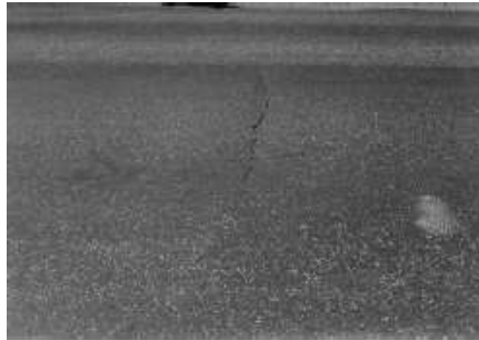
FIG. X1.28 Low-Severity Longitudinal and Transverse Cracking
