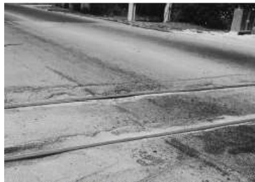
FIG. X1.39 Medium-Severity Railroad Crossing
