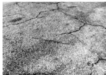
FIG. X1.9 High-Severity Block Cracking
