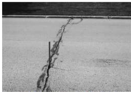
FIG. X1.29 Medium-Severity Longitudinal and Transverse Cracking
