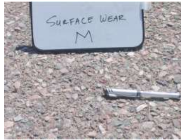
FIG. X1.54 Medium-Severity Weathering (Surface Wear)
