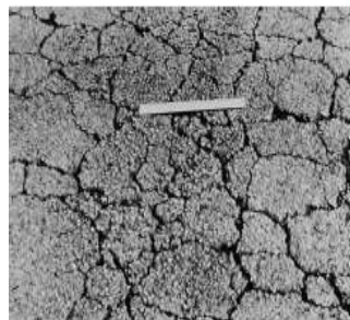
FIG. X1.3 High-Severity Alligator Cracking
