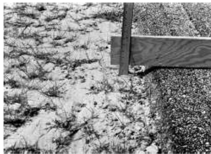
FIG. X1.25 Low-Severity Lane/Shoulder Drop-Off
