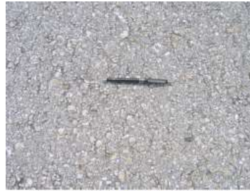
FIG. X1.53 Low-Severity Weathering (Surface Wear)
