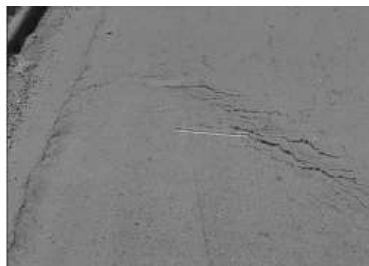
FIG. X1.48 Medium-Severity Slippage Cracking
