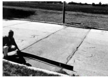
FIG. X1.32 Medium-Severity Patching and Utility Cut Patching
