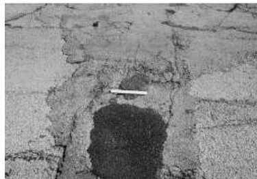
FIG. X1.33 High-Severity Patching and Utility Cut Patching
