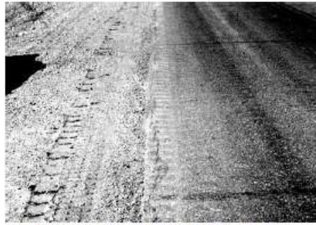
FIG. X1.22 Low-Severity Joint Reflection Cracking
