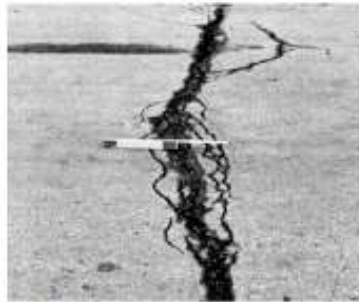
FIG. X1.24 High-Severity Joint Reflection Cracking
