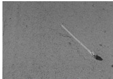
FIG. X1.47 Low-Severity Slippage Cracking
