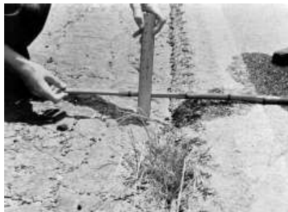
FIG. X1.26 Medium-Severity Lane/Shoulder Drop-Off
