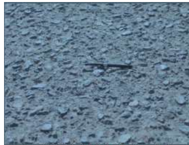
FIG. X1.55 High-Severity Weathering (Surface Wear)
