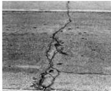
FIG. X1.23 Medium-Severity Joint Reflection Cracking
