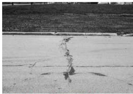
FIG. X1.30 High-Severity Longitudinal and Transverse Cracking
