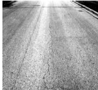
FIG. X1.1 Low-Severity Alligator Cracking
