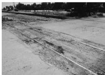
FIG. X1.40 High-Severity Railroad Crossing
